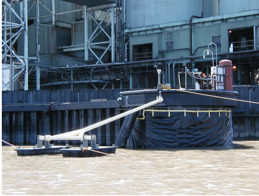
Figure 13. The North End Cell, just before the AFB is attached. The mooring cell is wrapped with the impermeable material providing an end seal for the system, and equipped with a Gunderboom-designed and manufactured bridging arm to support the floating system, and air supply equipment that will provide the system with pressurized air for automatic cleaning.
