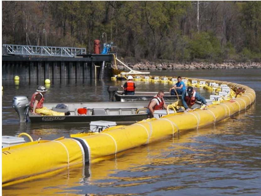
Figure 26a. The installation team members attaching the control boxes to the AFB and installing the air line hoses. Special attention must be paid to securing all of the cables and lines.
