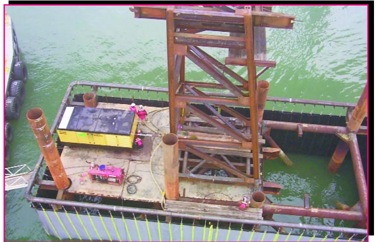
The layout of the compressor, manifold and air lines.
