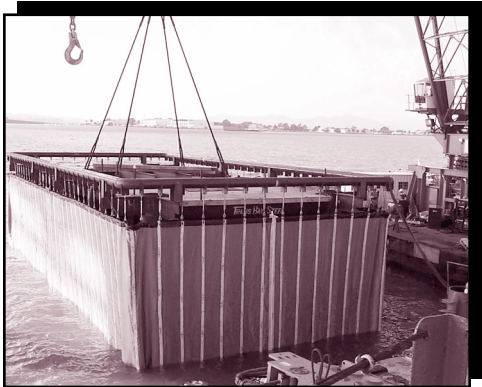
The curtain and template are lowered into position over the pin/locator pile.
