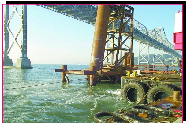
This is the template that was in use for the first two pilings, with no attenuation and then with the standard air bubbler curtain.
