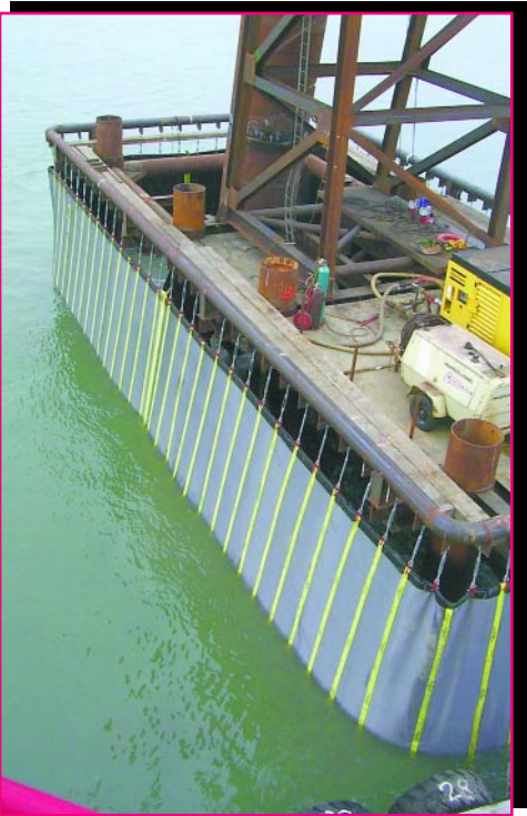
The sound attenuation curtain bulging during operation.
