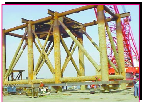
The template was taken to the staging facility so the curtain could be installed.
